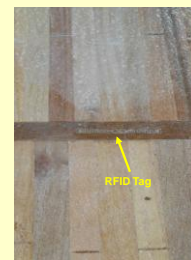
RFID in Timber Door
